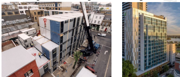
(Murray Grove project building in London, U.K., and the Ibis Hotel East Perth building in Australia)
